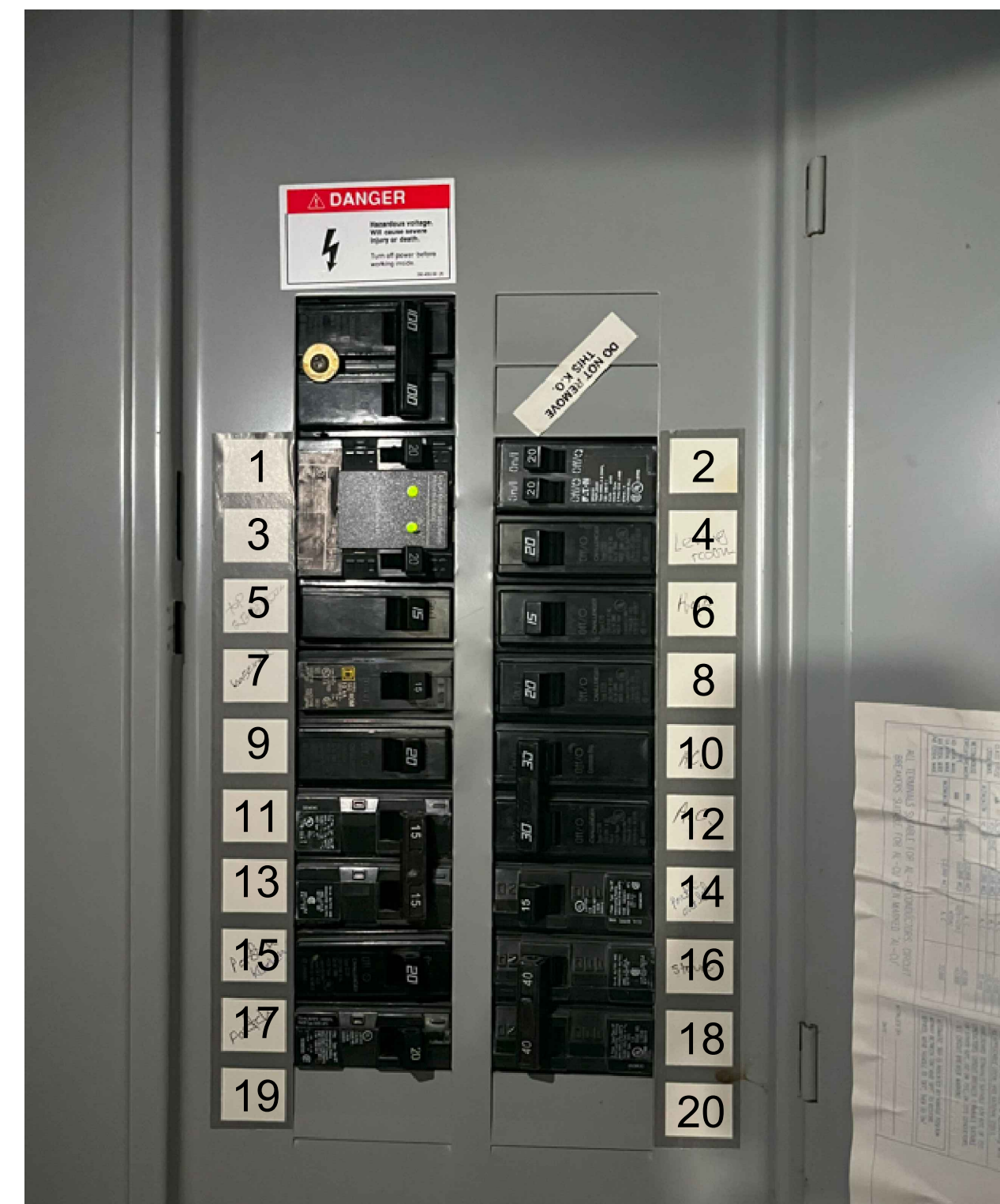
existing electrical panel image
